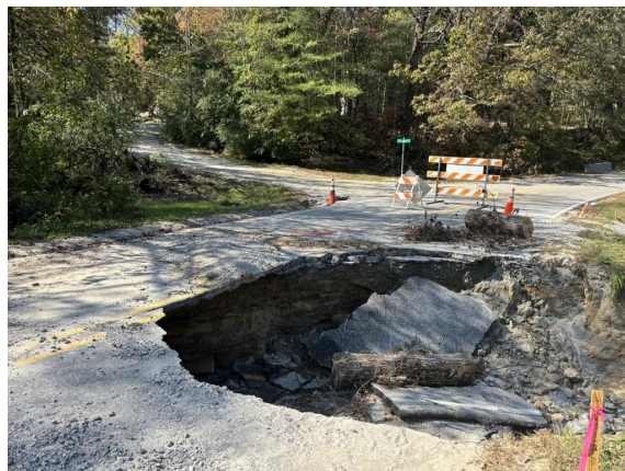
Sinkhole over a culvert in Edneyville, NC
